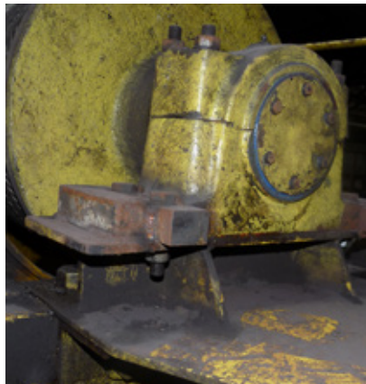
Plummer Block Prior to Retrofit
